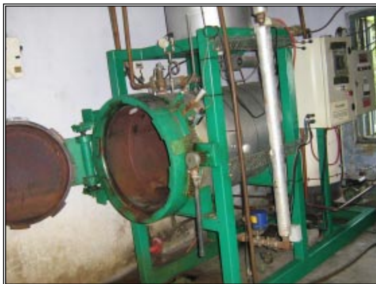
Autoclave installed at JNM Hospital-Kalyani under WBHSDP, Health Department, Government of West Bengal for treatment of non-anatomical bio-medical waste
