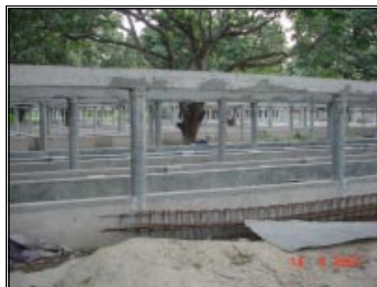
Construction of Vermi compost pits for the Model Facility Project in North Dum Dum and New Barrackpore municipal areas
